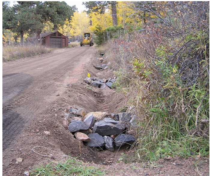
Figure 9: Rock check dams in a small ditch ( www.casfm.org/stormwater_committee/LID-Summary.htm )
