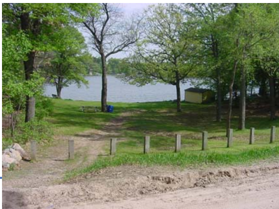
A swale is excavated to catch runoff from the boat ramp and parking lot (June 2001)
