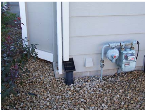
The downspouts outlet into perforated drain tile leading to the new rain garden (August 2004)
