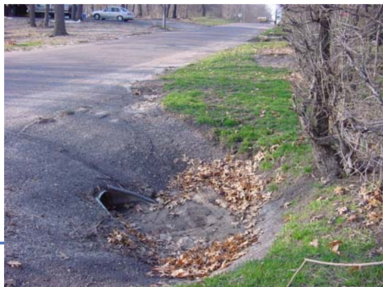
A culvert directs water through the Aymar property into Coon Lake. The buffer is designed to intercept this flow (April 2002)
